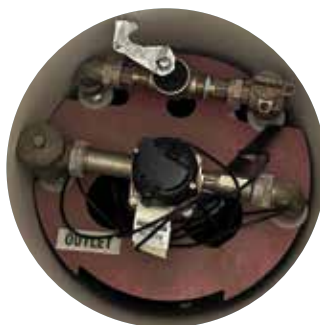
Meter Pit (inside)
